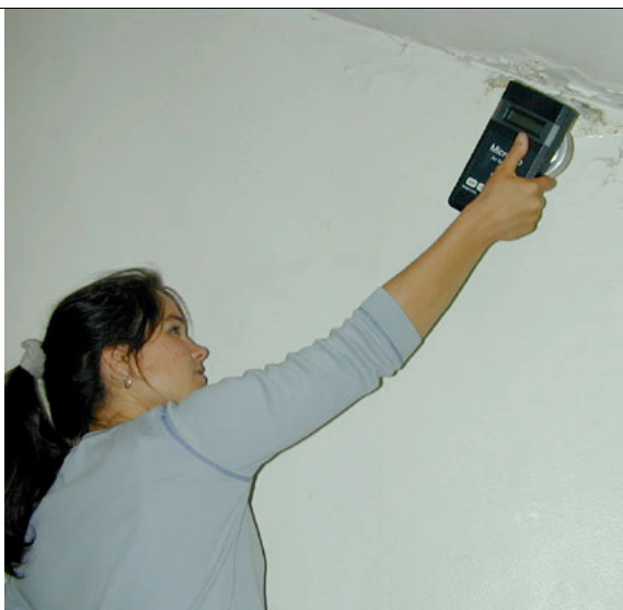
a) Collecting from a water damaged area
