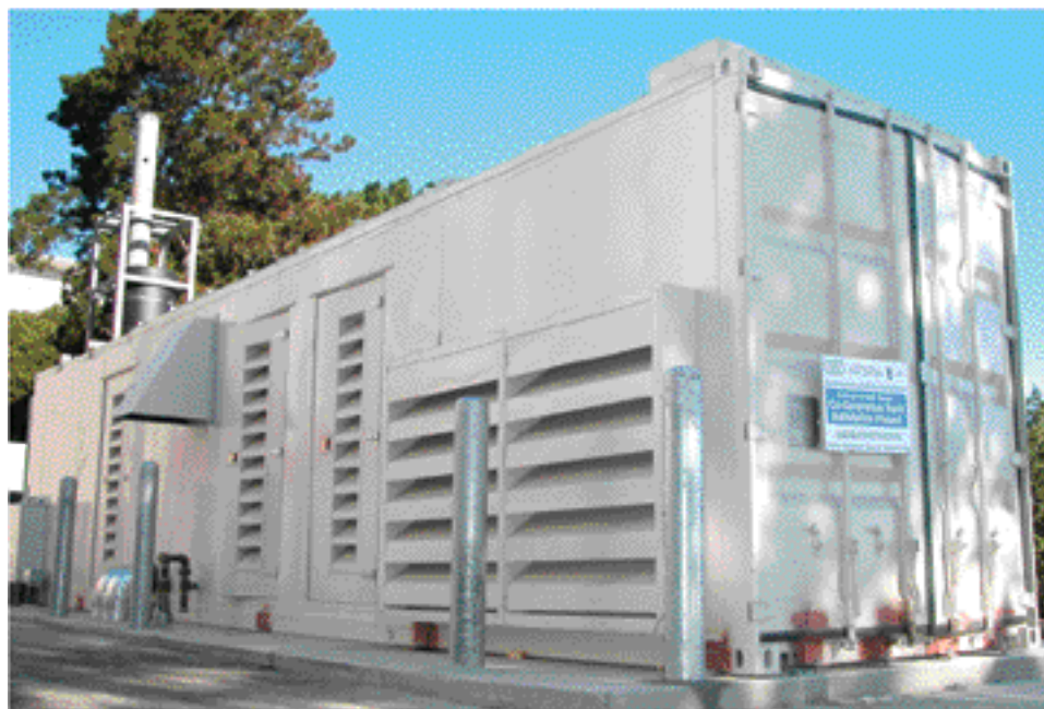
Soundproof enclosure for CSM's cogeneration system
